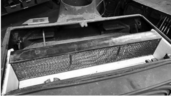
Fig. 23. Lift combustor from the chamber.
