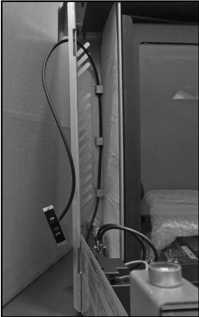
Figure 82: Pre-installed ON OFF switch SIT assembly.
