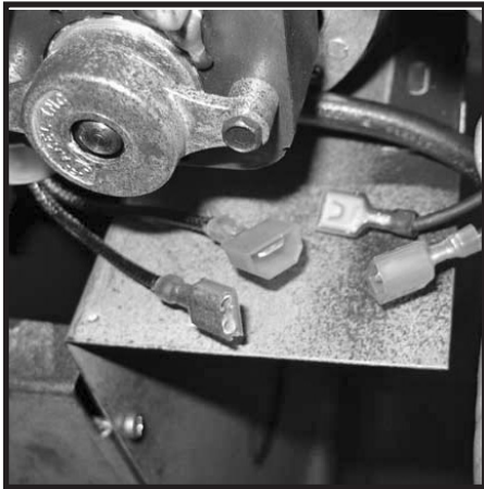
Figure 15: Disconnecting fan wires.
